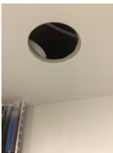
CCTV & riser cupboard
