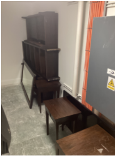
Main electrical intake cupboard
