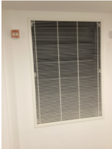
AOV in basement level
