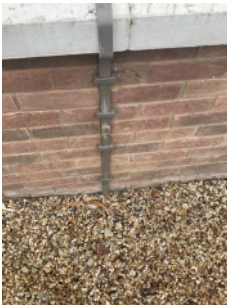
Lightning protection system
